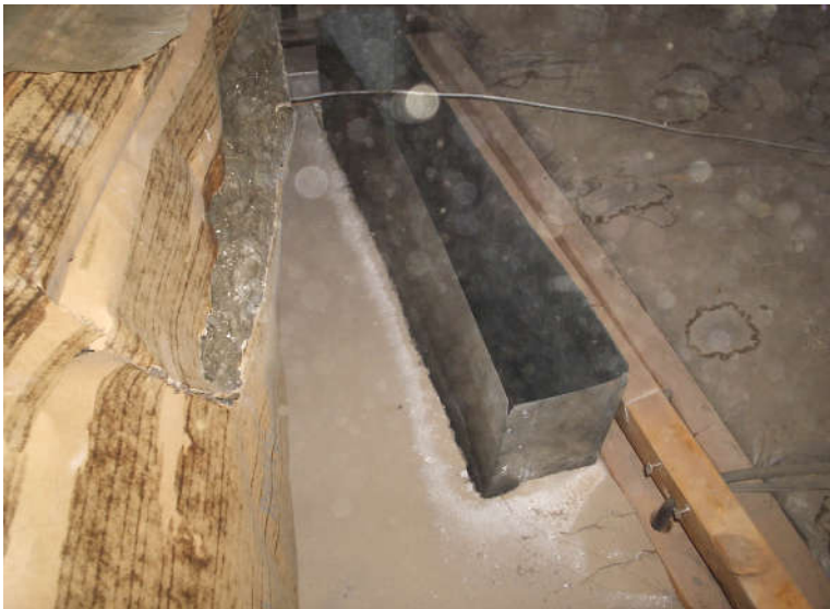
11 The combustion air vent is partially blocked by insulation in the attic space.
